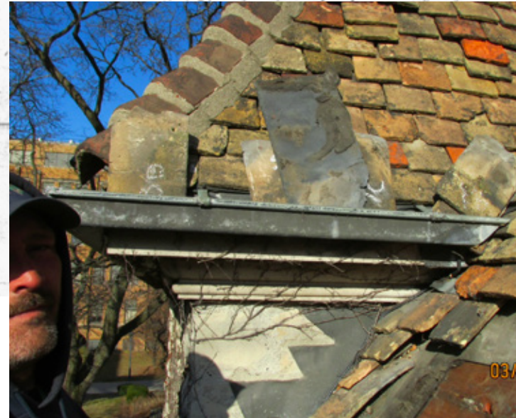
A preliminary roof tile inspection was conducted at the lower west corner on the south slope of the nave.
