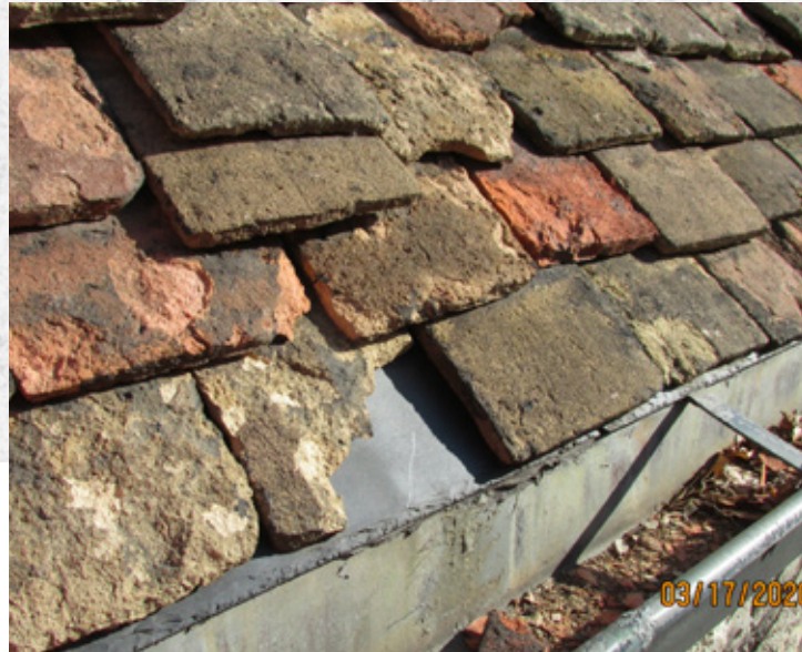
Approximately 25 - 30% of the historic clay roof tiles are deteriorated and would not survive removal and reuse.
