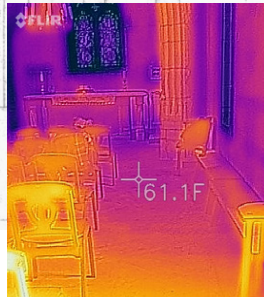
Thermal infrared camera image reveals temperature gradient caused by failed radiant floor heating system in the Chapel nave.
