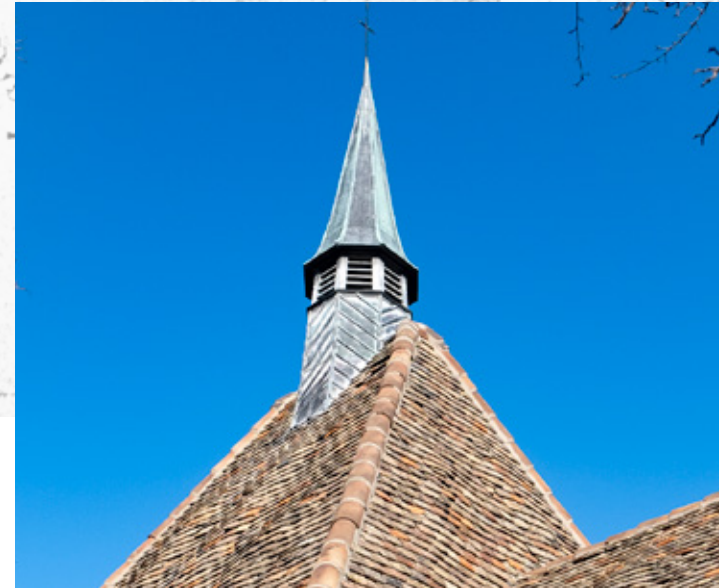
Solder joints and copper roofing of the historic are in need of repair and reinforcement. The solid roof deck and closed floor of the louvered area need opening for installation of the ventilation shaft.
