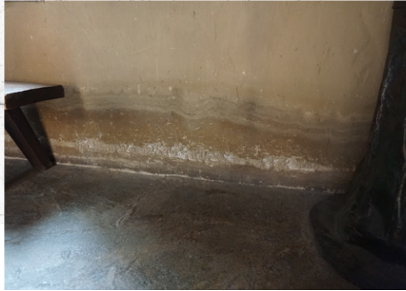
Rising damp is visible at the base of the interior wall resulting from moisture introduced by landscape plantings and mulch beds at the perimeter of the chapel.
