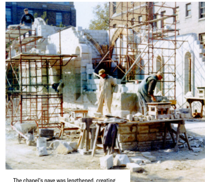
The chapel's nave was lengthened, creating additional space inside for larger worship services and gatherings.
