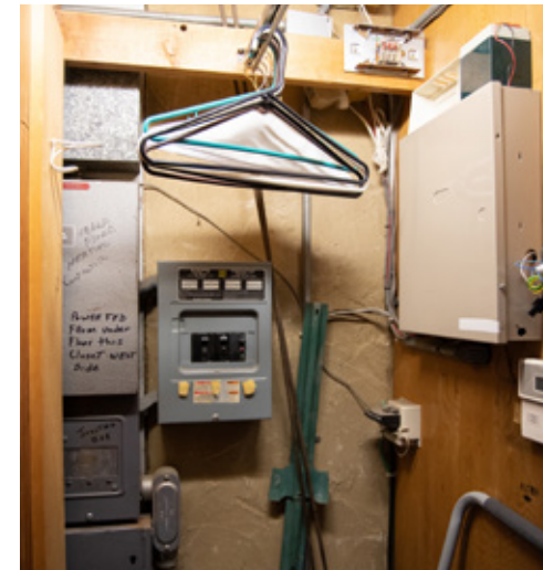
Existing electrical boxes are crowded into the sacristy closet and need upgrades.
