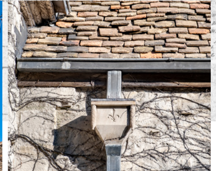
Gutters and downspouts are also in need of improvement to adequately drain water away from the chapel walls and foundation.
